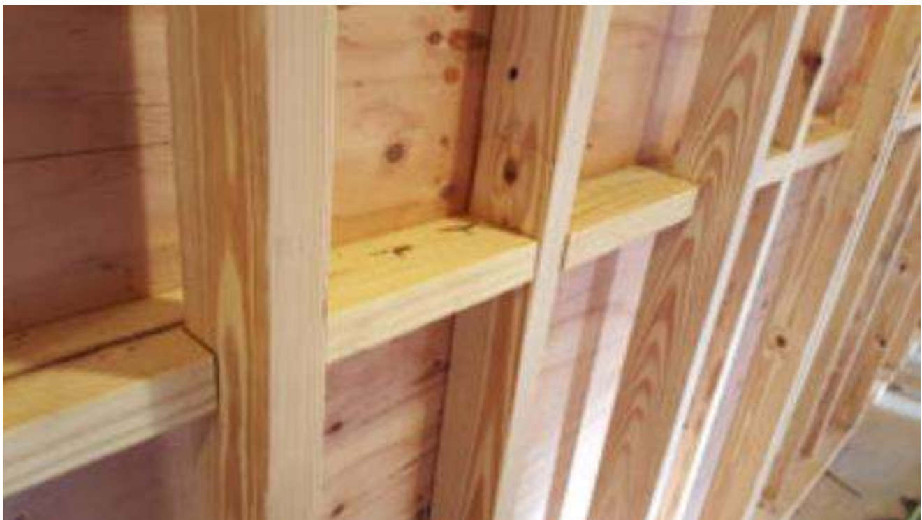
Blocking between studs in an exterior wall to support the horizontal joints in the plywood sheathing
