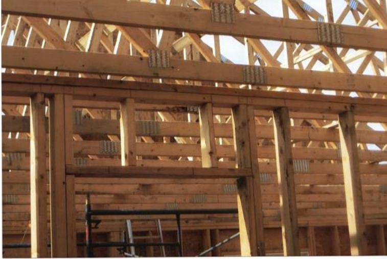
Unsupported interior partitions. Furring strips should be added before interior partition are attached.
