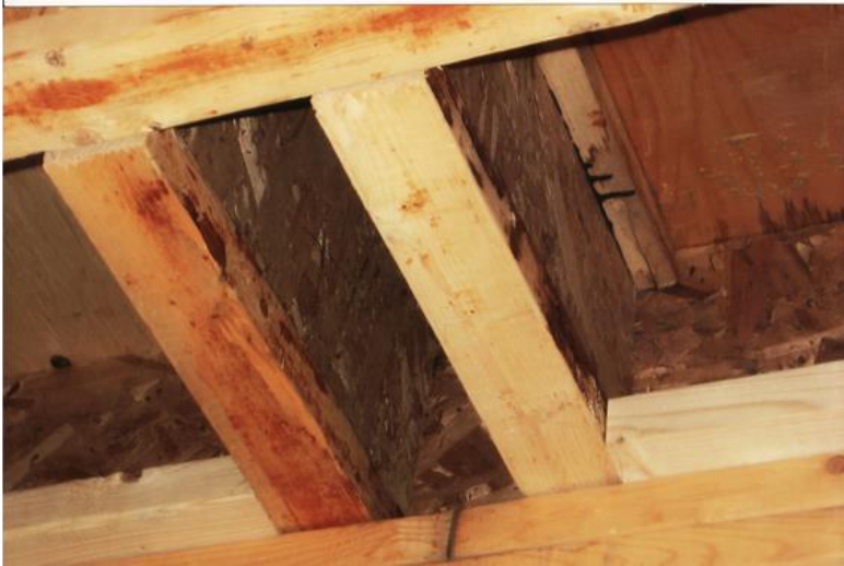
Rim joist missing and improper framing
