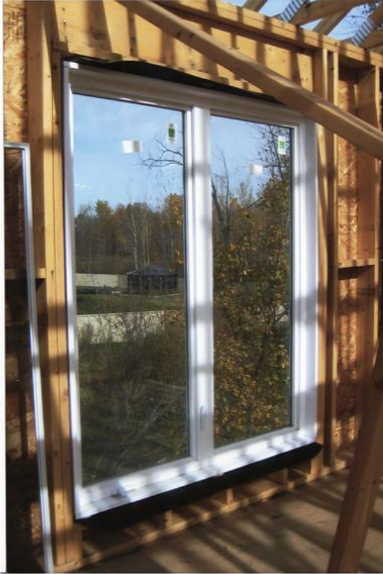
Bottom of window very low and concern for person falling out the second floor
